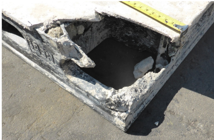
29.40 Profile corner torn out
