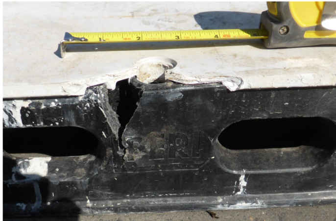
29.39 Anchor hole torn out
