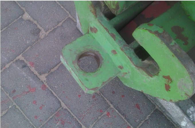
13.10.16 Head Bolt | Castle Nut missing
