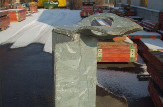
32.31 Crane eye bent
